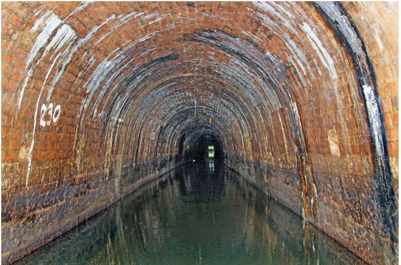
Looking east along the tunnel towards the portal in August 2016; the good condition of the brickwork is clearly seen. 230 painted on the wall indicates 230 metres from the portal. Photo John Lower
